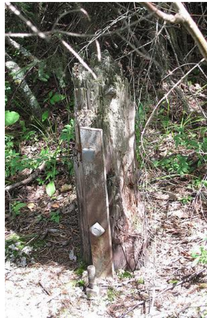
Bolts and Steel Anchored this Telephone Pole on the Bare Rock at Norway
