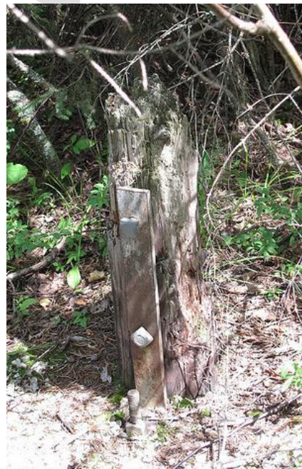
Bolts and Steel Anchored this Telephone Pole on the Bare Rock at Norway
