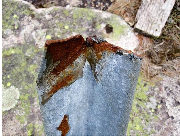
Burnt piece of steel from Sioux River tower. Result of explosive?
